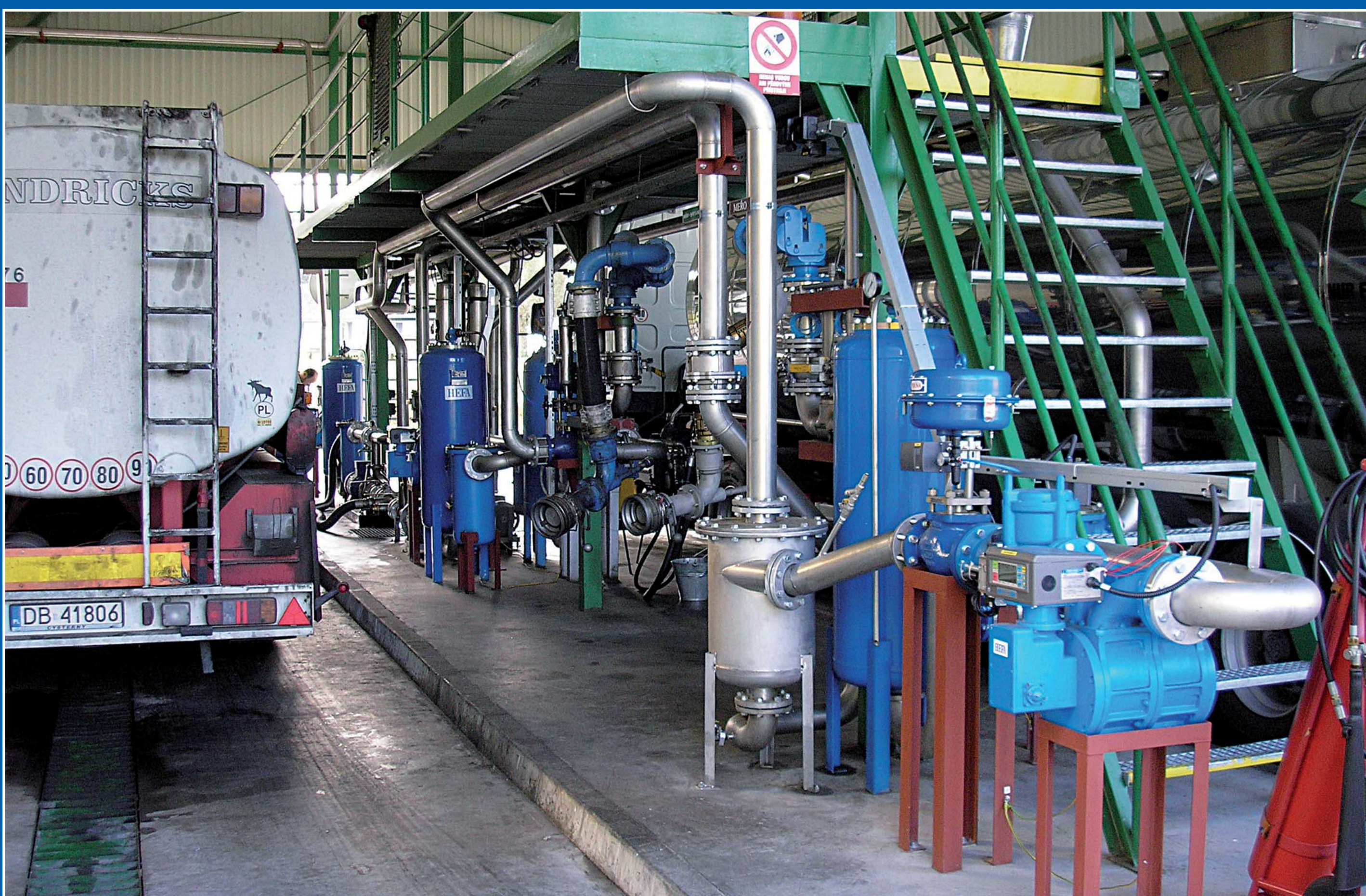
Top and bottom loading of fuel products
