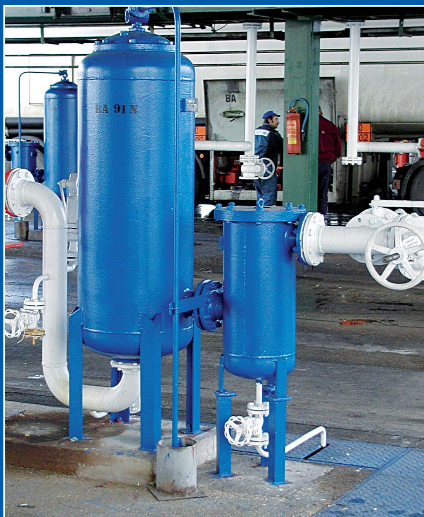
Air separator and filter
